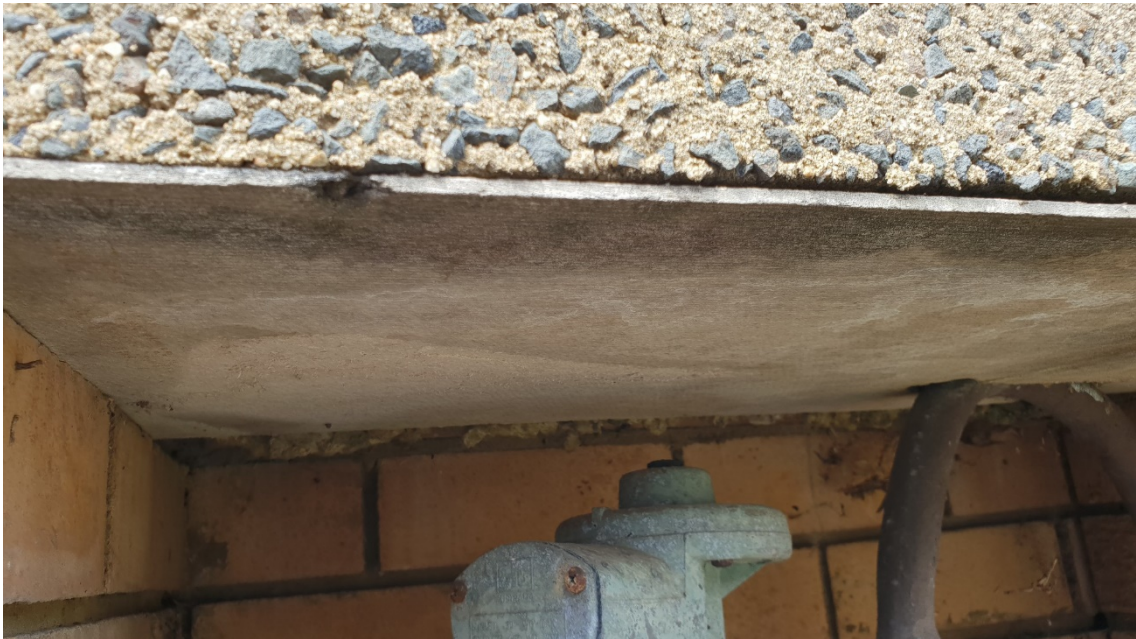
Photograph No. 8: Flat asbestos cement sheet substrate to concrete lid over gas meter at 71 Kerrs Road, Lidcombe
