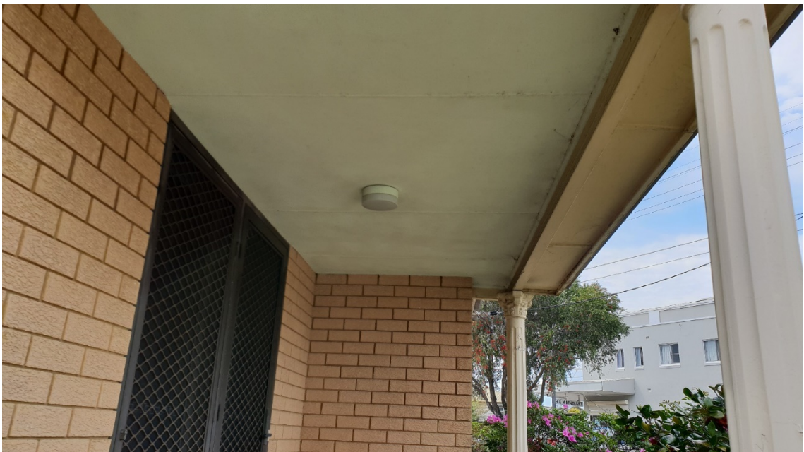
Photograph No. 6: Asbestos cement sheet soffit lining over the front verandah at 71 Kerrs Road, Lidcombe NSW
