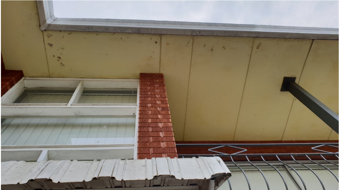
Photograph No. 1: Asbestos cement sheet eave and upper level verandah soffit lining on the front of the house at 65 Kerrs Road, Lidcombe NSW
