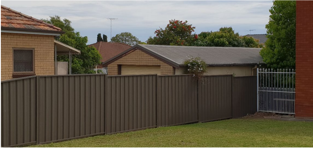
Photograph No. 7: Garage at 71 Kerrs Road, Lidcombe that has flat asbestos cement sheet wall cladding
