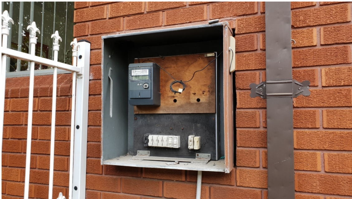
Photograph No. 3: Asbestos based 'Zelemite' electrical backing board in electrical meter cabinet at 65 Kerrs Road, Lidcombe NSW
